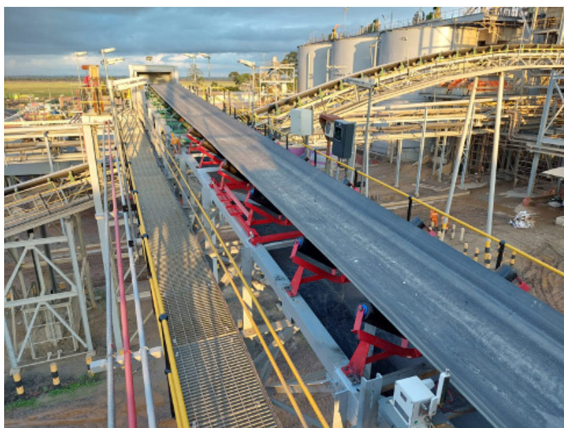
Sasco Belt Scale Installation in Ghana
