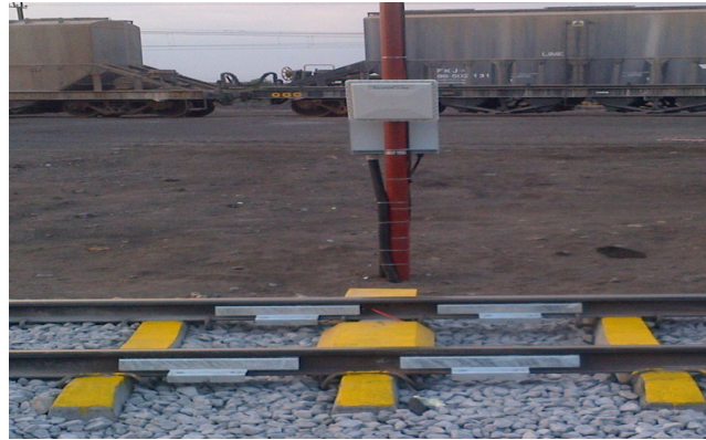
The RW-WIM model T04 installed with one automated vehicle identification readers.
